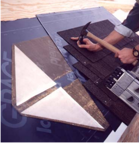
Illustration 2.55 Asphalt shingle roofing being installed over Z Mesh. Note sandwiching between “Ice and Water Shield”
