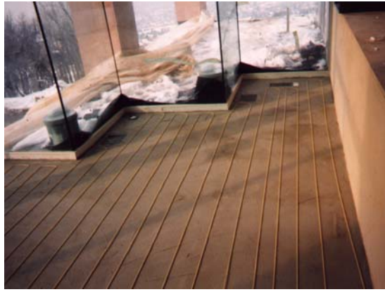
Illustration 2.13 Tuff Cable installed on top of mortar bed in space heating installation. Tuff Cable will be covered with thinset mortar prior to floor covering installation.
