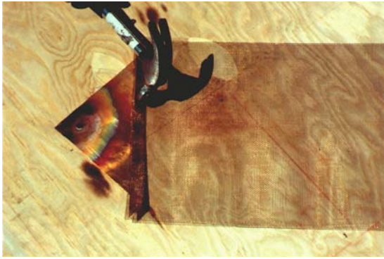
Illustration 2.47 Z Mesh inserted into fold of Transition Plate and fold flattened using hammer.
