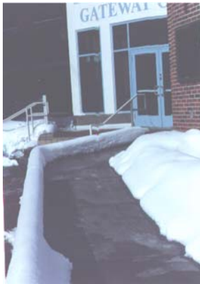
Snow melting of handicap ramp with Tuff Cable.
