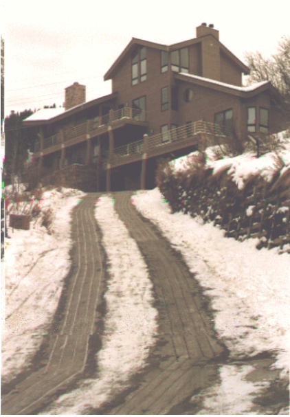
Illustration 2.20 Retrofit snow melting system installed in driveway
